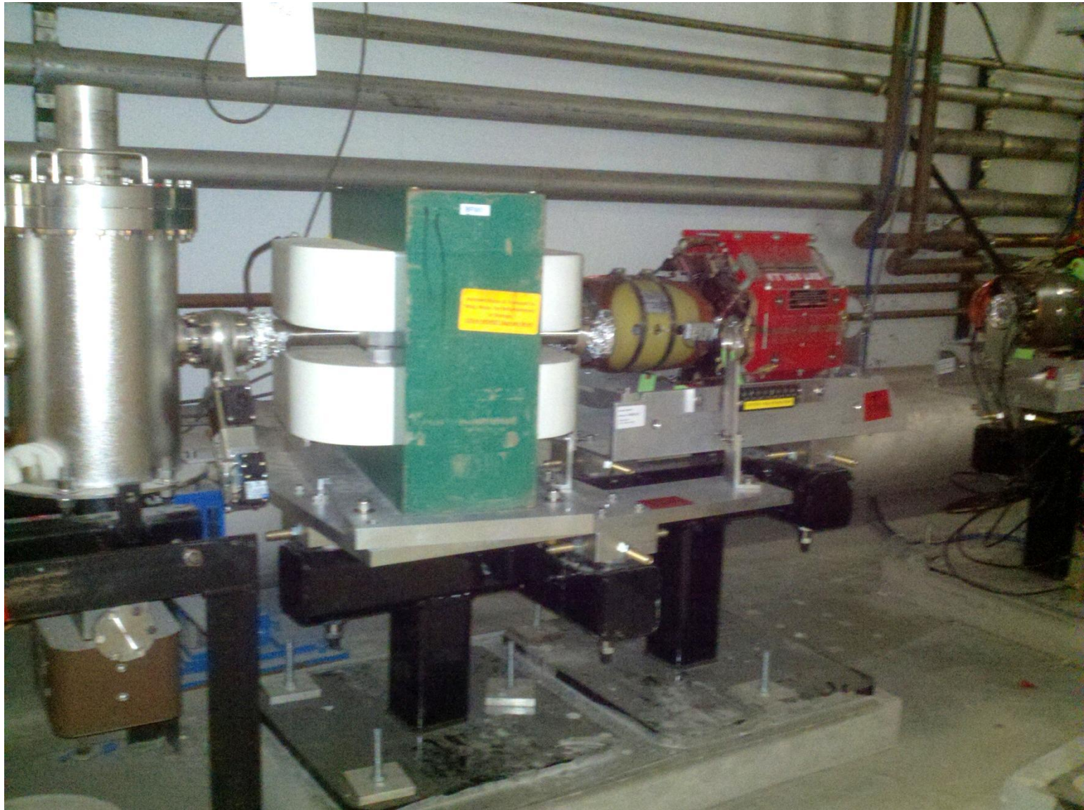
Spectrometer Dipole Installation
