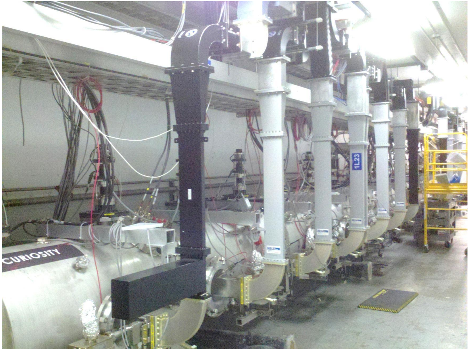
1L23 Waveguide Installation
