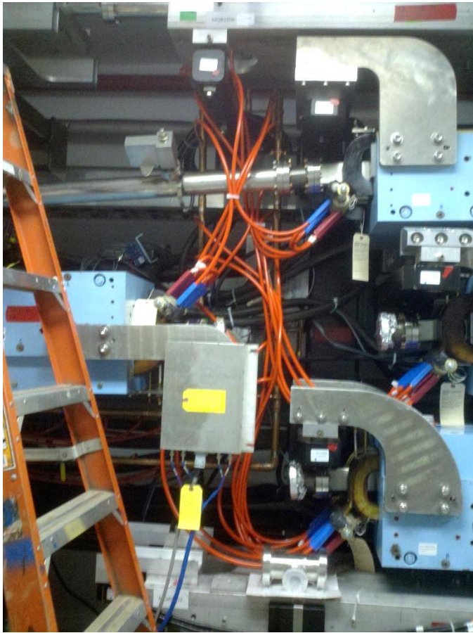
LCW Hose Installation
